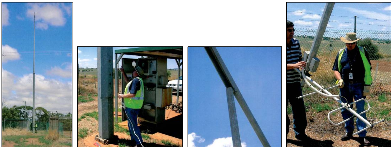
Example of a SCADA Antenna Tilt (hinged) Pole
