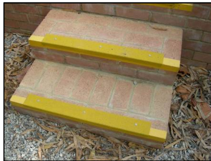
Example of a Non Slip Treatment on Edge of Brick Steps
