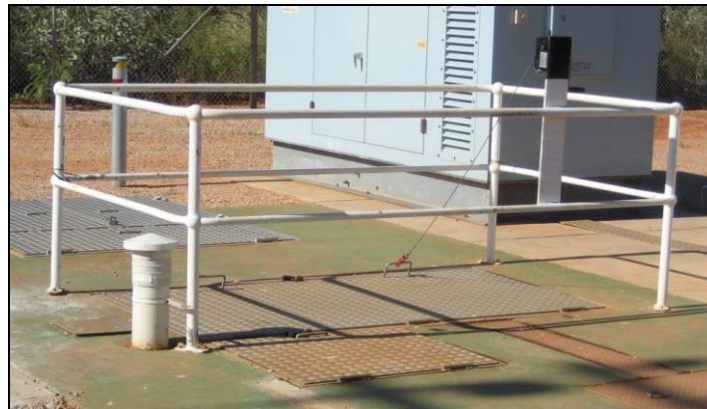
System for Hinged Covered Wet Well in Secured Submersible Pump Station Site
